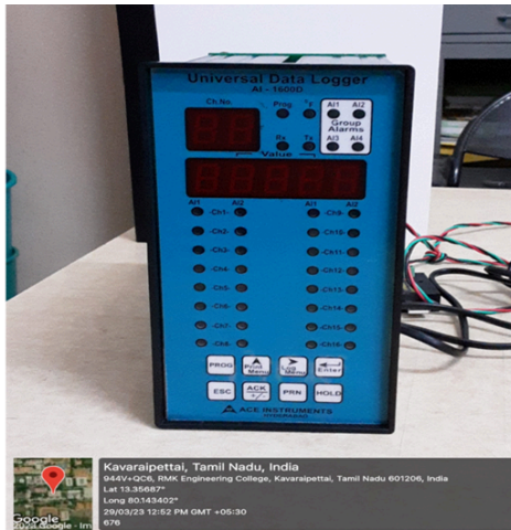
Data Acquisition System (16 Channel-microcontroller based temperature data logger- Model AA-1600D- RTDPT-100/4-20mA for Pressure, stress and strain transmitter)
