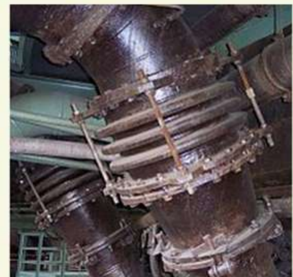
Stainless steel pipe expansion joint, with control rods.
